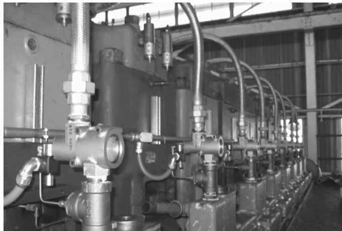
Cam actuated start valves with pressure-actuated in-head check valves
